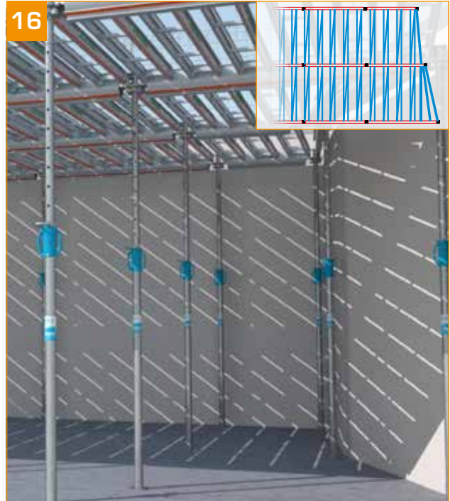
- Adjust the level using a laser level, ST by ST. - A gauge stick hanging from the formwork allows laser adjustment to be performed by one person. - Conduct a final head locking check at this stage.
