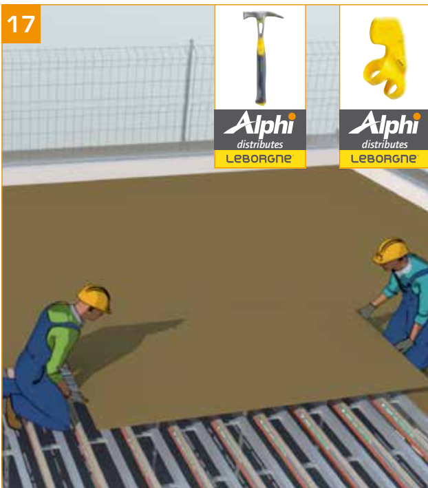
- When the structure is finished and the height has been adjusted: lay the plywood. - Use the plywood cutting support (see Accessories p. 9-10). → Peripheral safety (skin, girder, etc.) ensured beforehand. → Use of the plywood cutting support.
